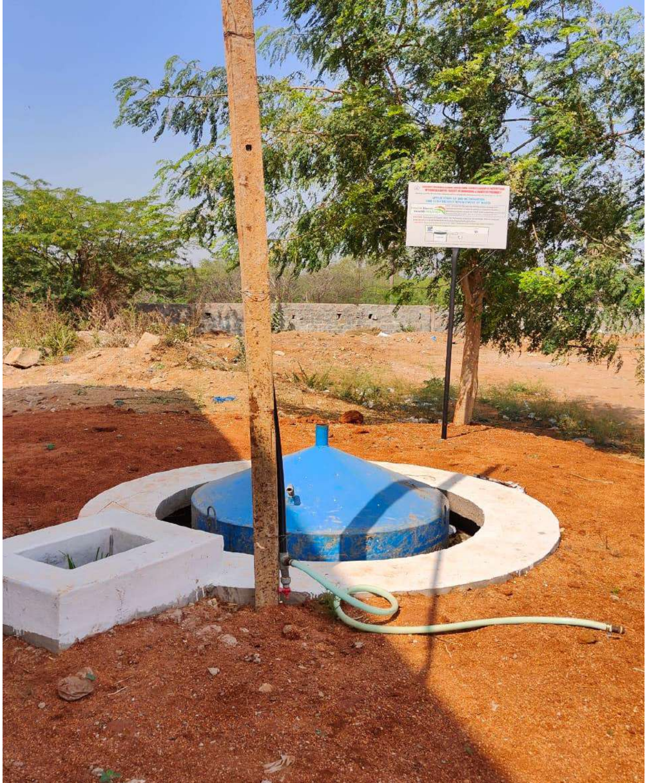
Bio-Gas Facility at Campus Premises
